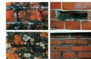
DAMAGE ATLAS CLASSIFICATION AND ANALYSIS OF DAMAGE PATTERNS FOUND IN BRICK MASONRY
